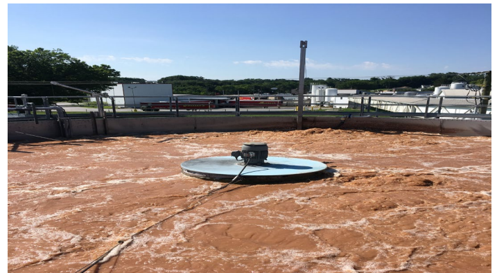
Figure 2. SBR tank processing high-strength dairy wastewater.
