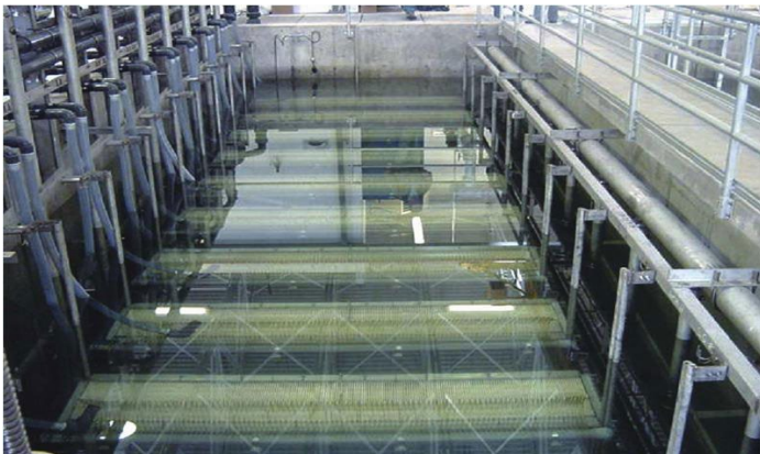
Figure 1. Fully installed and operating Kubota MBR system. https://www.kubota.com/products/solutions/
