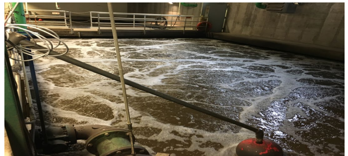
Figure 1. MWTP aeration basin after PBII treatment, showing normal foam development.
