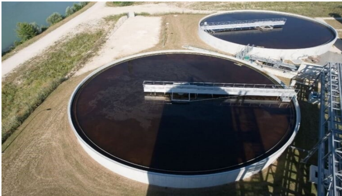
Figure 1. A small mechanical plant with primary and secondary clarifiers similar to the National Park mechanical system.
