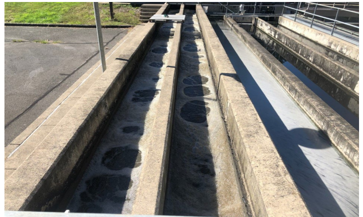
Figure 1. 0.2 MGD activated sludge plant oxidation ditch biological treatment supported by applications of ProBiotic Scrubber® II and Candy Carbon®.
